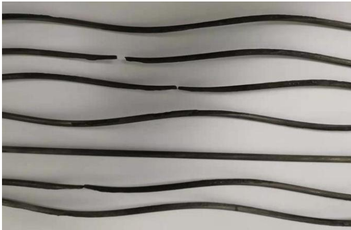
Fig. 2.7 Disassembled corroded steel wires
