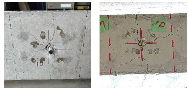
(a) 拡底 60 No.10 (割裂破壊) (b) 拡張 60 No.10 (割裂破壊)
